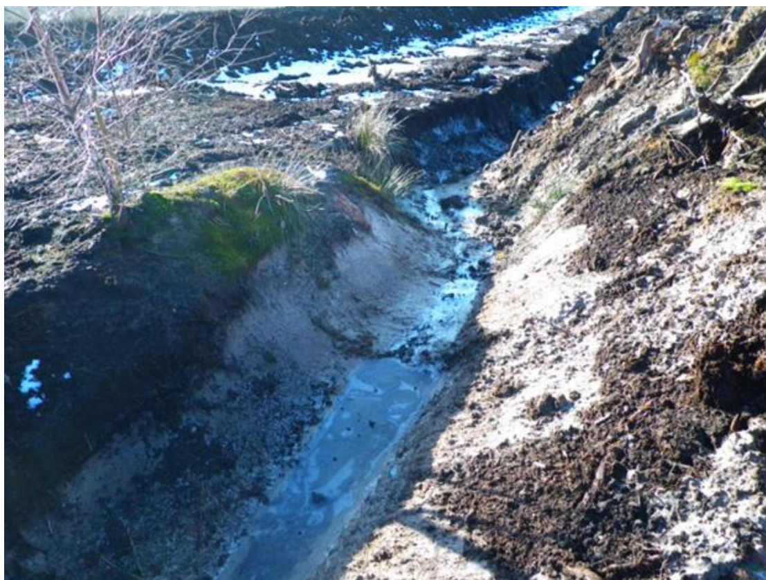
Figure 5 Exposed and eroding sand deposits below peat in the north east corner of peat extraction area (photo taken January 2015 reproduced from report No SHF.1633.001 with permission of Newgate Kennels Ltd)
