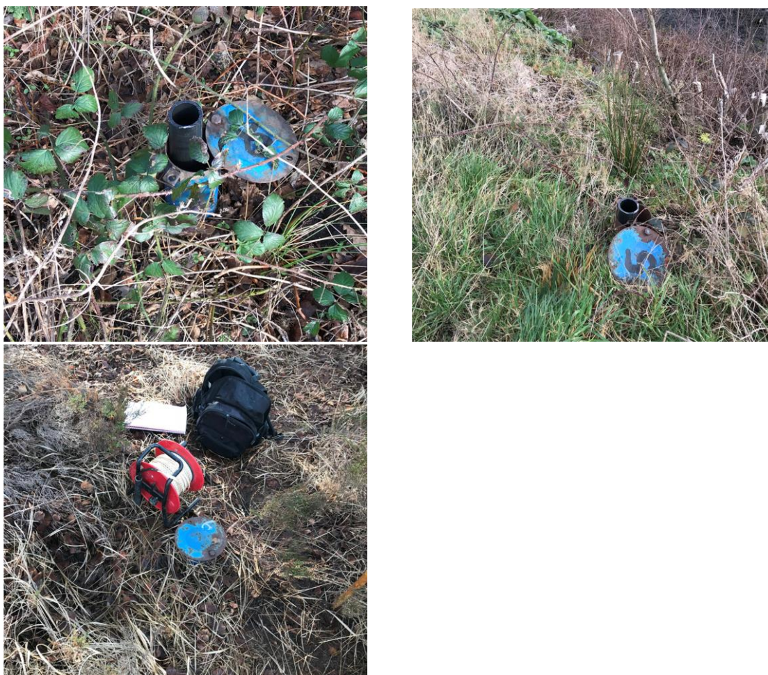
Figure 13 Effects of ground lowering on monitoring well datum at 08/07, 05/07 and 06/07, Peat Extraction area
